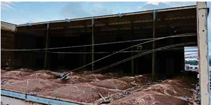
Figure 13, 14: Sentral Building 4 - Before HSE initiative
